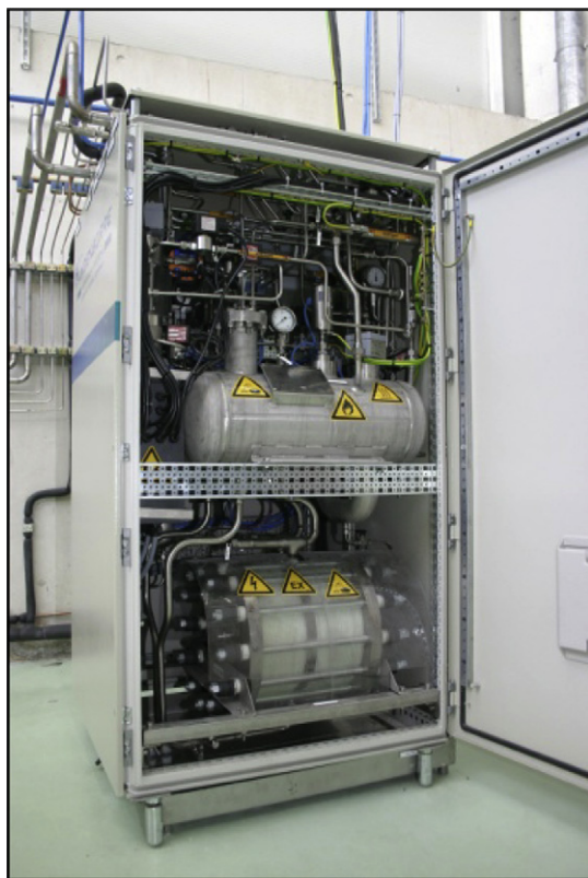
FIGURE 14.15 Interior view of the alkaline electrolyzer, model H2 IGEN 300/1/25, manufactured by the company Vandenberg (now named Hydrogenics). (For color version of this figure, the reader is referred to the online version of this book.)
